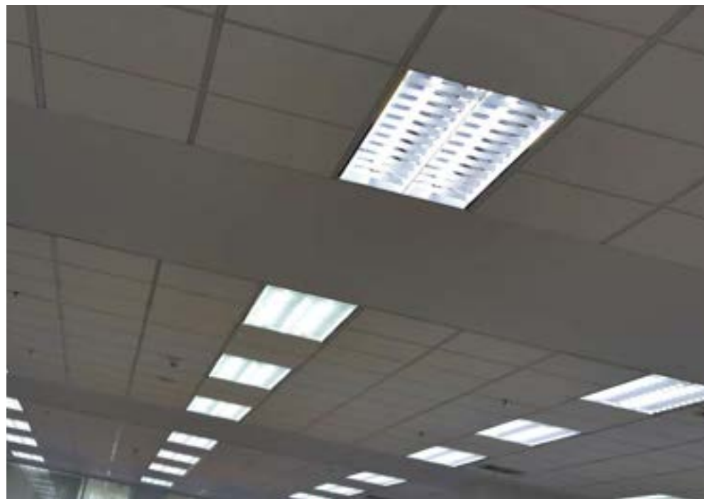
Figure 3.25. Fluorescent light fixtures in an office setting.
